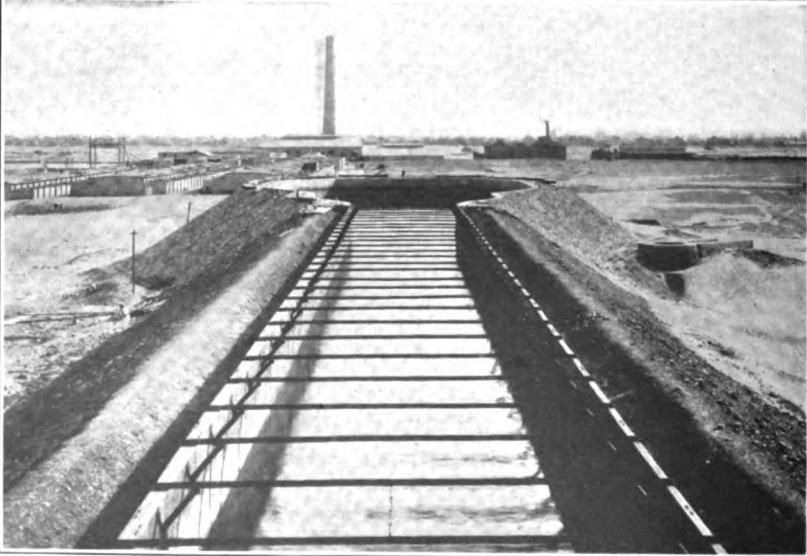
SLUICE GATES, SERVICE RESERVOIR, AND PART OF THE STEEL CANAL, WADI KÔM-OMBO IRRIGATION SCHEME.
