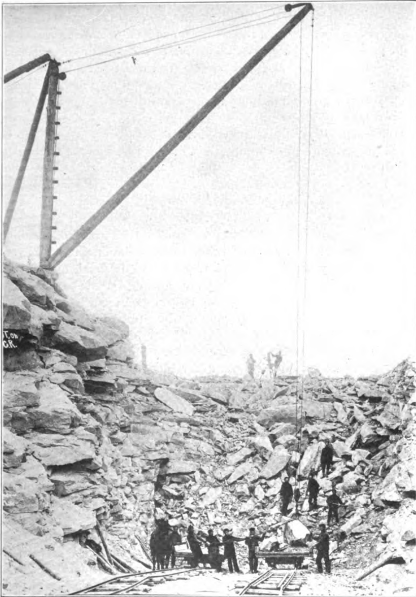
A DERRICK FOR LOADING BLASTED ROCK ONTO CARS. DRILL AT WORK IN THE BACKGROUND.
